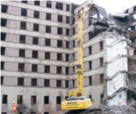
Approximately 95% of the material from the demolition of the old Vancouver Hospital Nurses' Residence is being recycled
